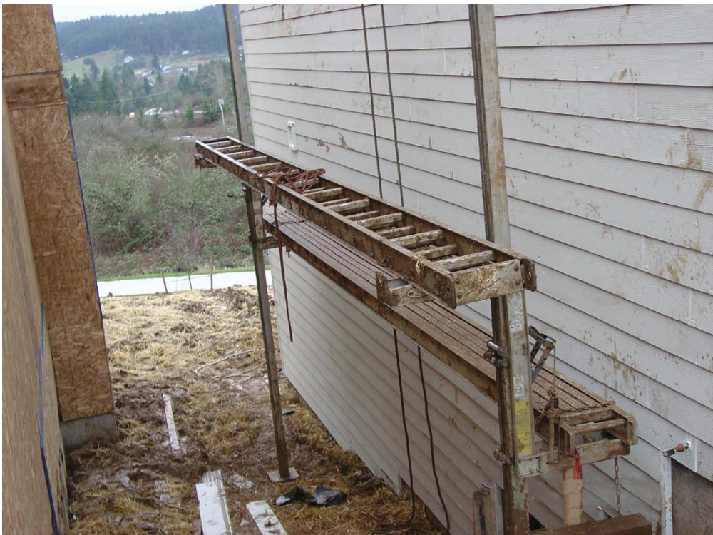
Pump Jack Scaffolds will normally have a work bench that can act as a top rail if it is 38 to 45 inches. Don't forget a midrail and guarding the ends – both are missing in this picture.
